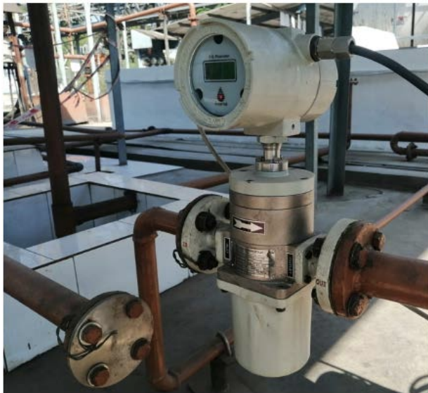
Distribution network PD meter (Unit 04 Power House)
